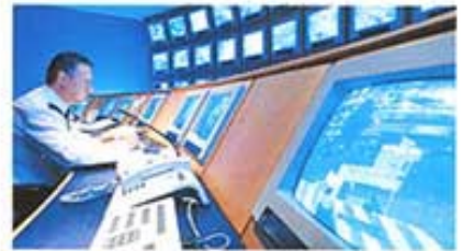
Favoured in systems such as CCTV where data security, capacity and suitability for ATA arrays is a requirement
